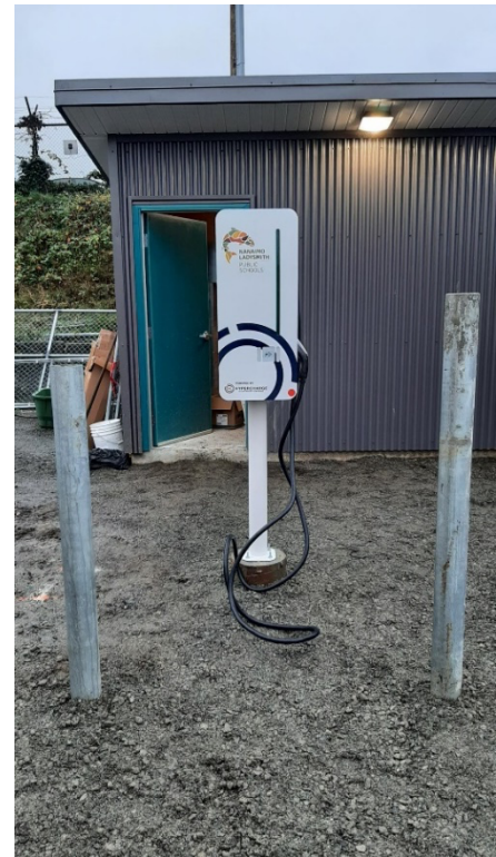
Figure 12. Charging infrastructure at SD 68
