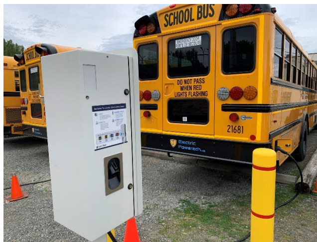
Figure 4. Electric school buses at School District 68, Nanaimo-Ladysmith. The District has purchased four electric school buses to date, and is committed to growing its fleet.
